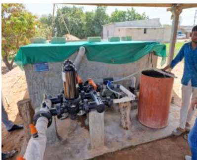
Pumps transport groundwater to the distributors of the drip irrigation hoses. Liquid fertilizer can be added.
